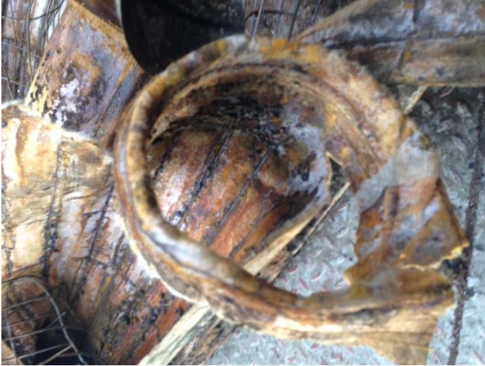
BAD BAGS PULLED FROM # 3 DUST COLLECTOR
