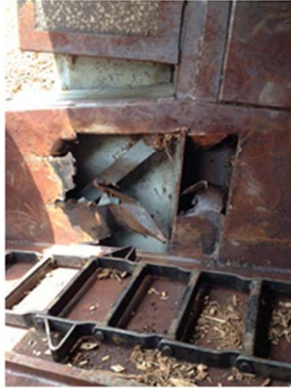
#2 Underpile worn through
